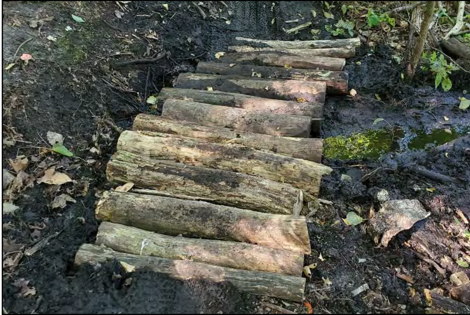
Photo 9. Corduroy crossing that needs to be replaced with a bridge.
