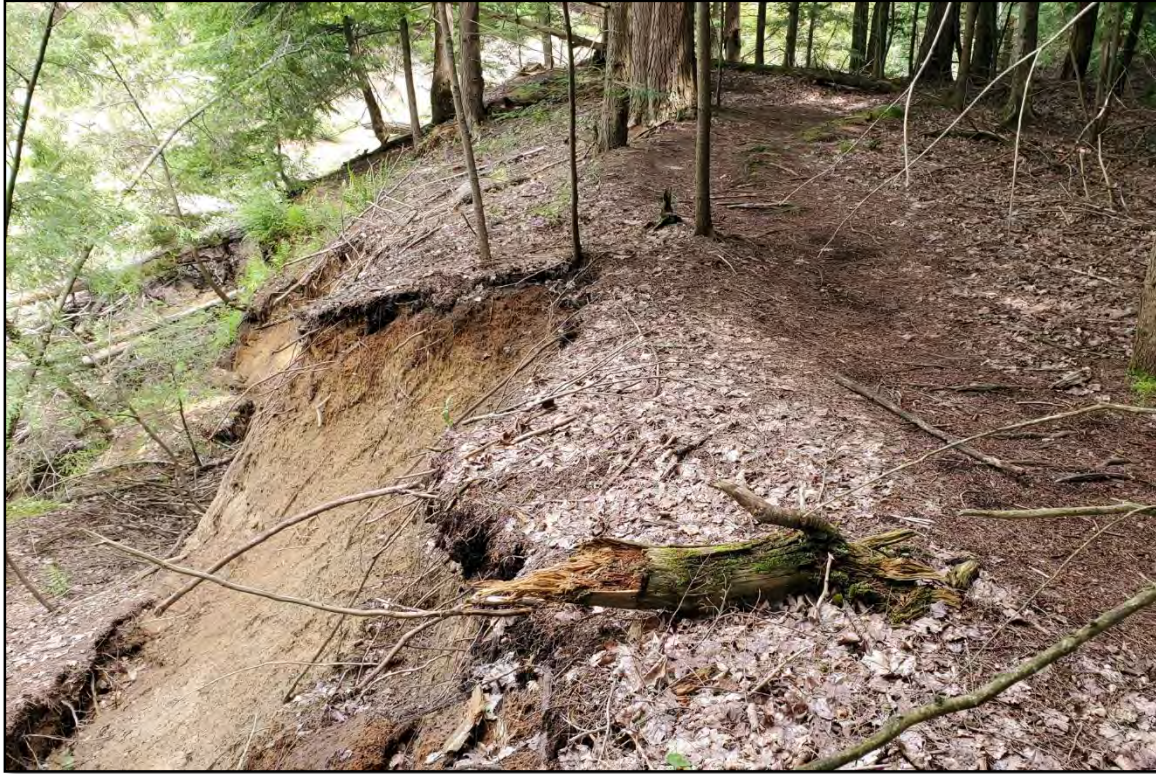
Picture 3. Trail close to slumping bank at the pond washout area; set back may be required.
